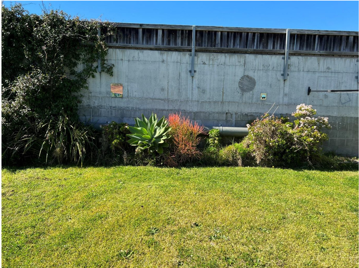
Figure 3c. Eastern boundary wall with a pipe, as seen from the southern portion of the Site. Photo taken 17 Aug 2023.
